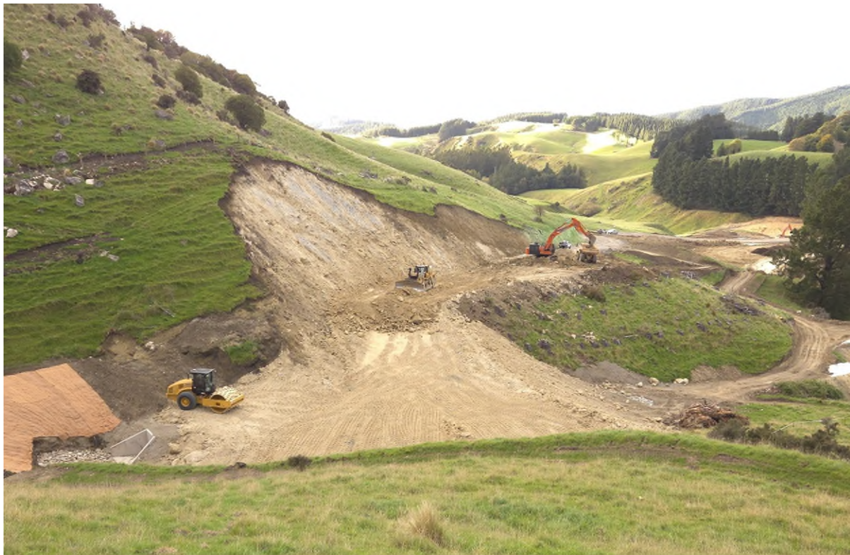
Figure 3: Steep slopes above and below the access road
