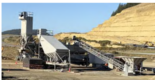
Concrete batching plant at Transwaste
